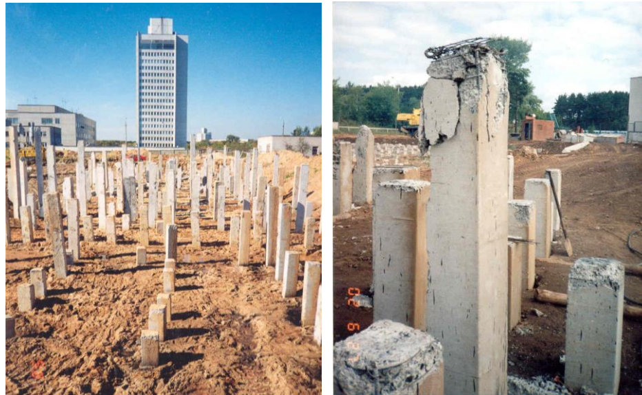
Fig.1. Piles not submerged to the design depths
