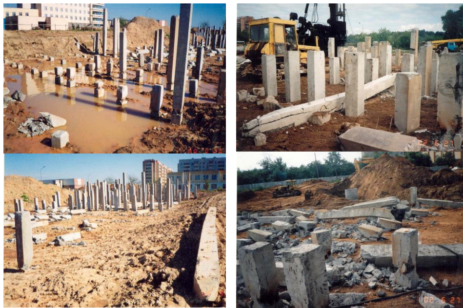
Fig. 2. Piles not submerged to the design depths
